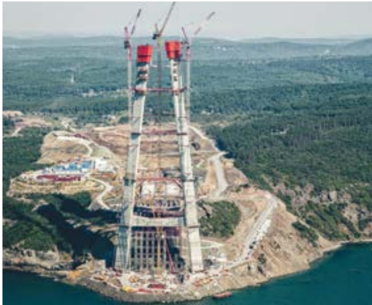
Connecting Asia and Europe, Turkey's transportation alternatives and commercial capacity will increase with the 3 rd bridge.
